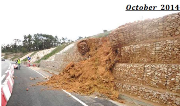
Figure 5. Damage to the gabion wall [11].
