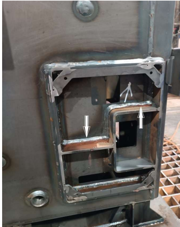
Figure 8. Passage of water through the welds on the box
