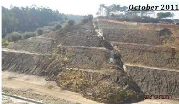
Figure 3. Occurrence of the first landslide during construction work [11].
