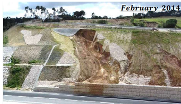
Figure 4. Sliding due to heavy rain [11].
