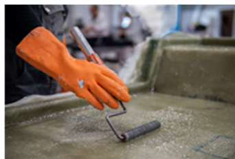
Figure 10. An example of manual lamination (hand lamination), application of the mixture with a roller.
