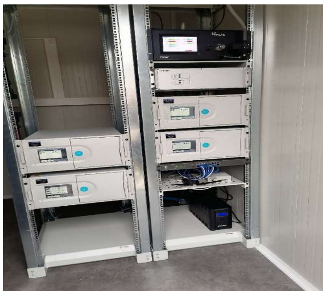
Figure 1. Interior of the Air Quality Measuring Station (author Hana Demirović).
