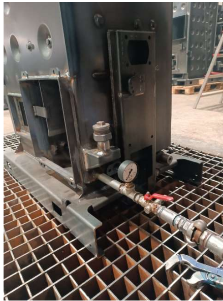
Figure 3. Setting the barometer at the lowest point of the boiler
